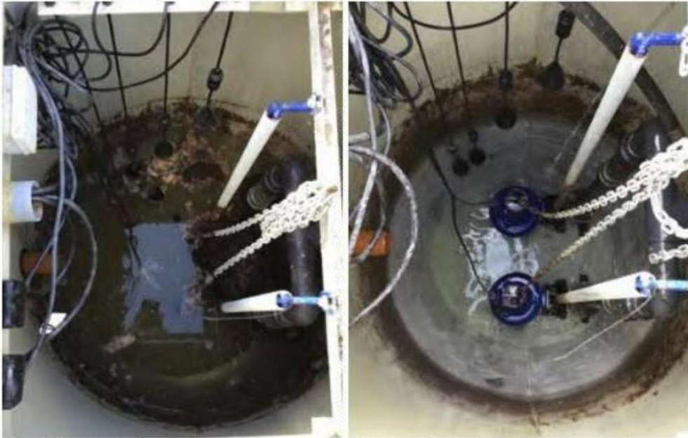
One of the blocked chambers
